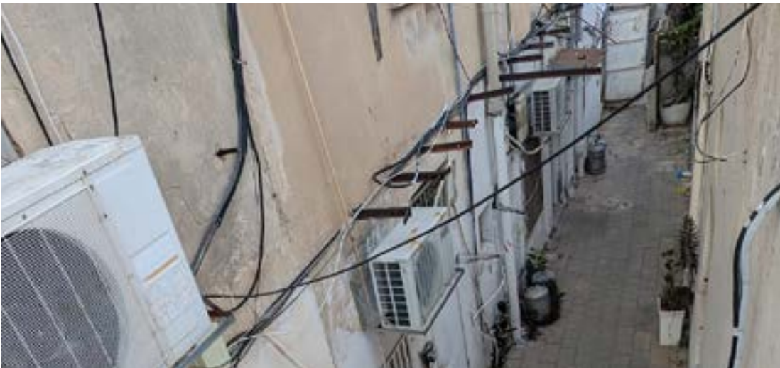
A dilapidated and overcrowded residential building in the Hatikva neighborhood. Photo: Neta Hamami Tabib
